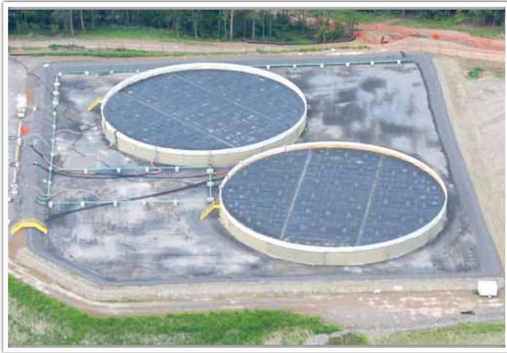
1 1/2 million gallon containments with floating roofs.
